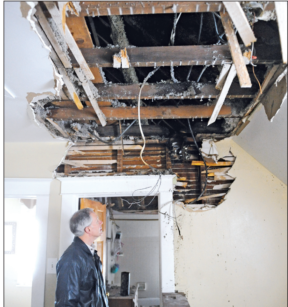
DAMAGE TO THE CEILING at the shelter operated by Advocates of Ozaukee was inspected Tuesday morning by Dave Fischer, a member of the non-profit agency’s board of directors. Photo by Sam Arendt
